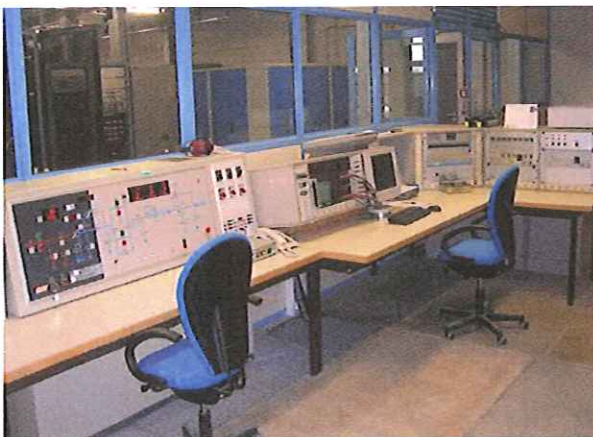
Control station for tests up to 15kA
